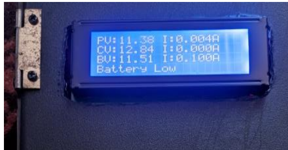
Gambar 6. Pengujian Under Voltage
